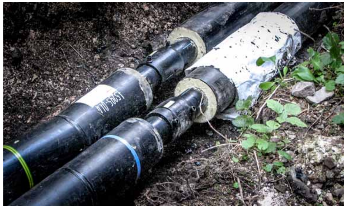
WORK // WATER PREINSULATED PIPELINE LOCATION // HIGH TATRAS MOUNTAIN - BELIANSKA CAVE
