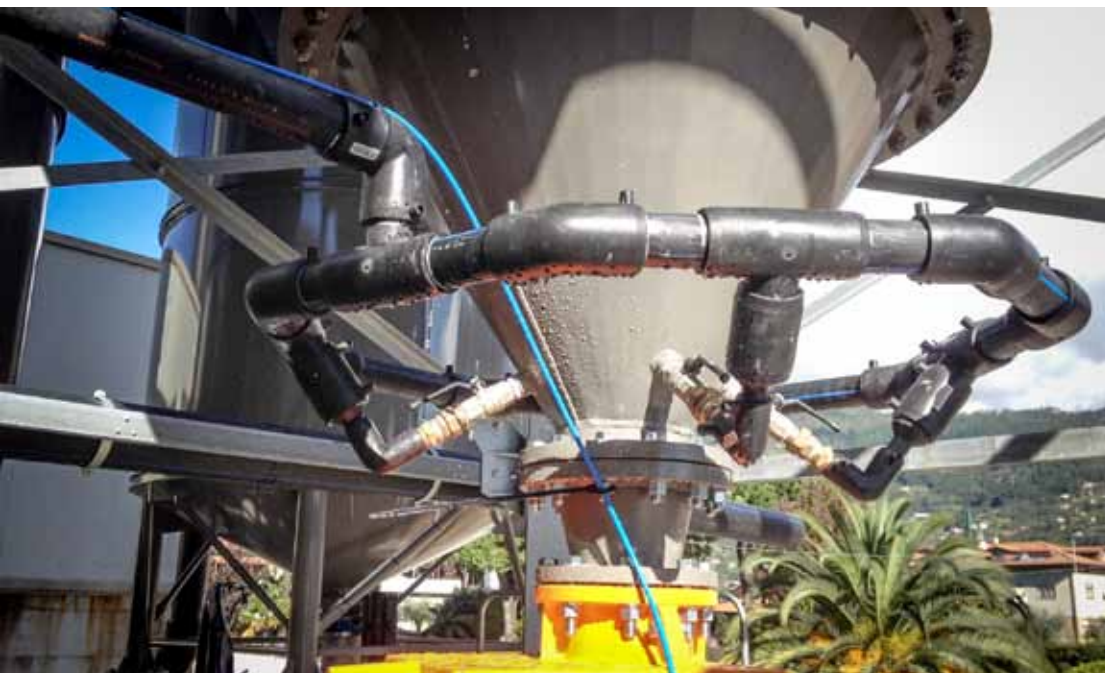
WORK // MARBLE QUARRY WATER TREATMENT PLANT LOCATION // MARINA DI PIETRASANTA - LUCCA
