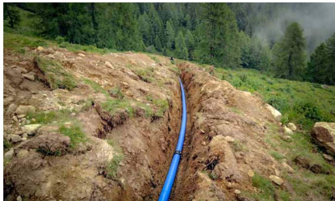
WORK // HYDROELECTRIC POWER PLANT LOCATION // VAL DI RABBI - TRENTO
