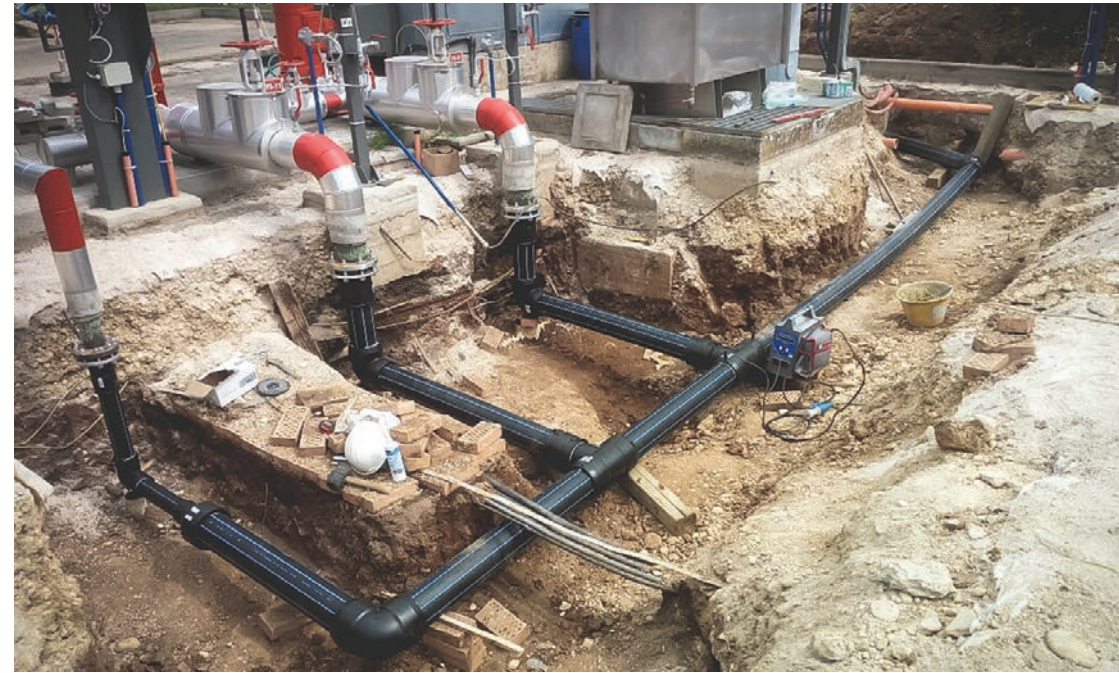
WORK // GAS DEPOSIT FIRE-FIGHTING PLANT LOCATION // GALLESE - VITERBO
