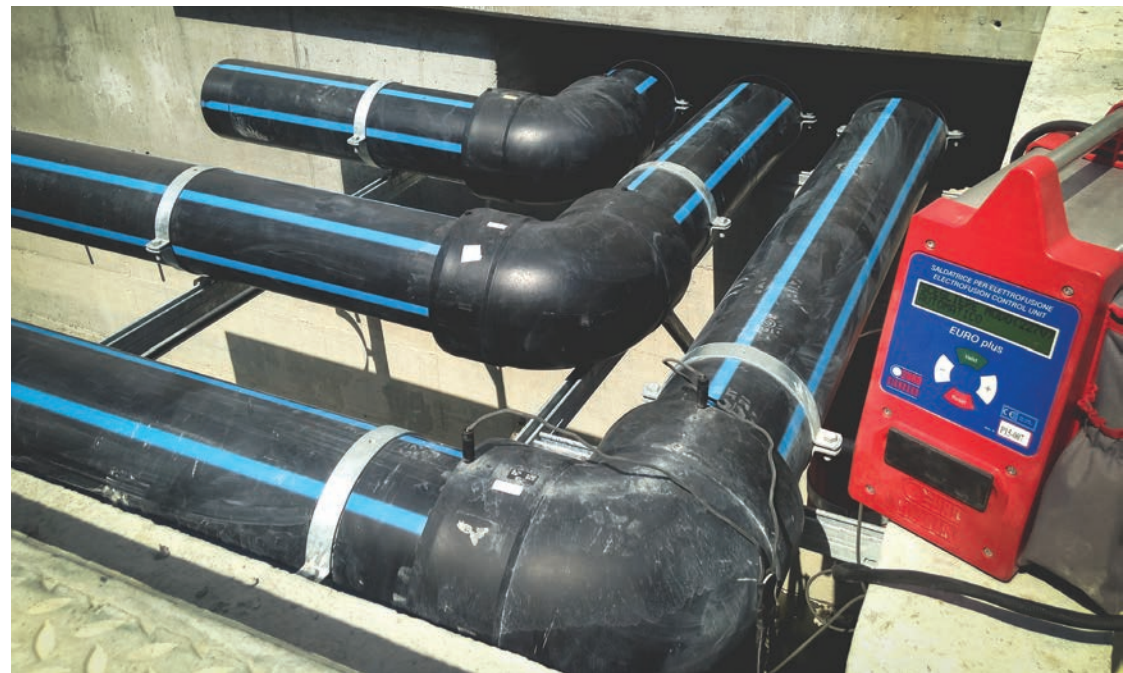
WORK // WATER PUMPING PLANT – RAILWAY STATION LOCATION // INDUNO OLONA – VARESE
